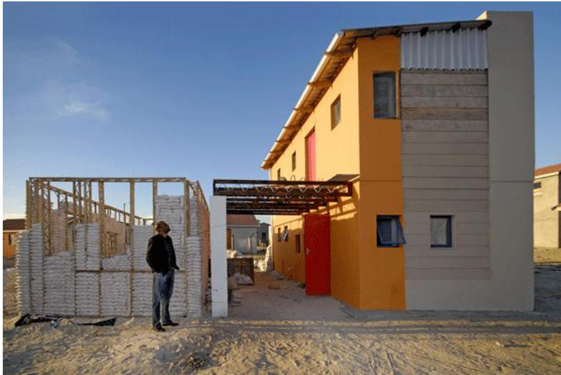
Picture 12 – Habitational building with one block under construction and other already done
